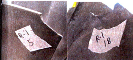
20 7F tip cracking
